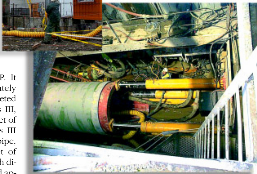
Around-the-clock deliveries of microtunnel pipe were required to allow pipe to be fed continuously into the jacking pits.
