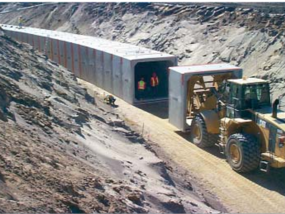
781 dry-cast concrete box sections were provided for the 4,777-foot long storm sewer in Phase I of the airport drainage system expansion.
