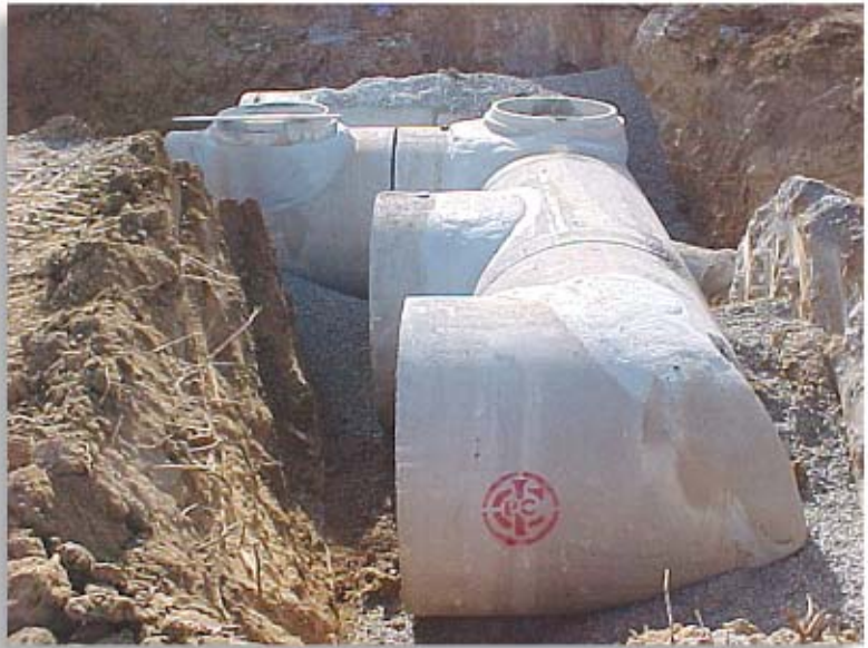
The system included 66-inch x 66-inch diameter 90° elbows and tees with four 72-foot runs of 66-inch diameter reinforced concrete pipe.
