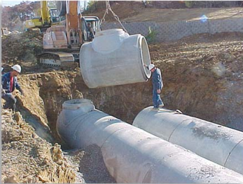
48-inch manhole tees with bulkheads were installed at the end of each 72-foot run to provide access to the Midland Manor Detention and Overflow System.
