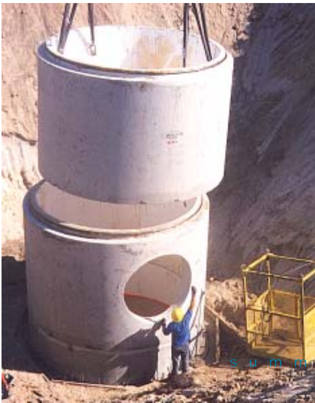
Workers position a section of 144-inch diameter RCP for a wet well lift station on the Buena Vista Trunk Sewer Project.
