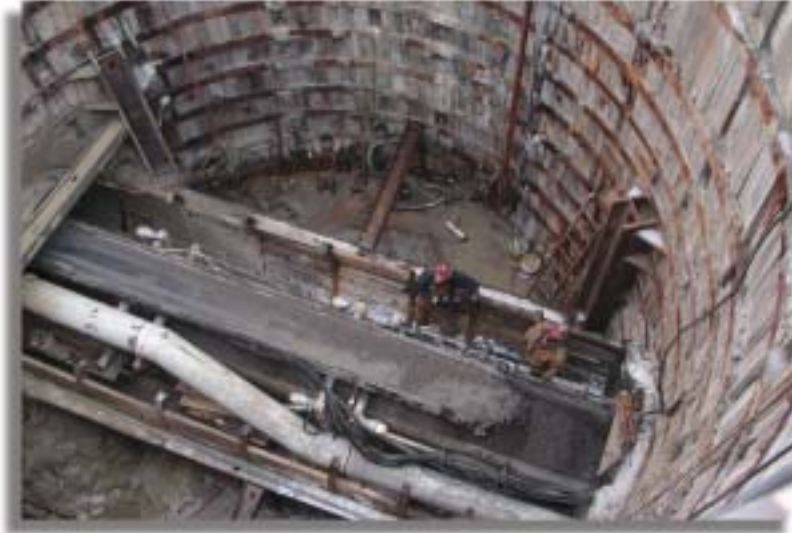
Excavated spoils being loaded and removed from construction pit following bore for 84-inch reinforced concrete pipe.
