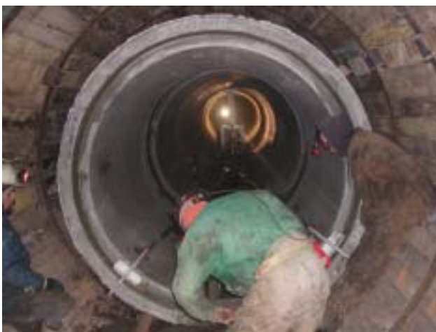
84-inch diameter reinforced concrete pipe being set inside of the steel rib and wood lagging sets as part of the bore and pipe jacking operation.
