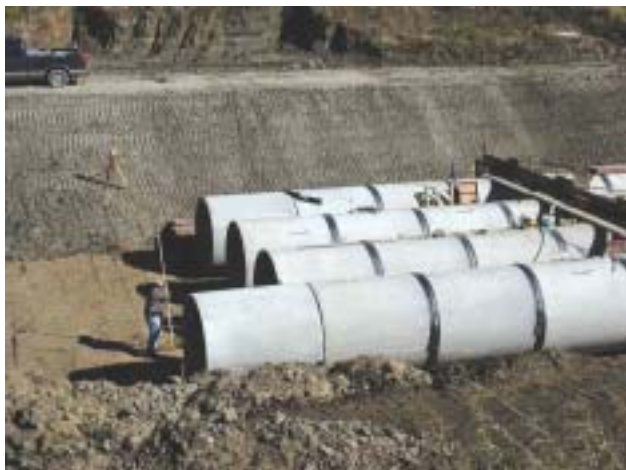
Frequent grade alignments and close joint tolerances help produce “rifle-barrel” smooth results inside the 72-inch reinforced concrete pipe culvert.
