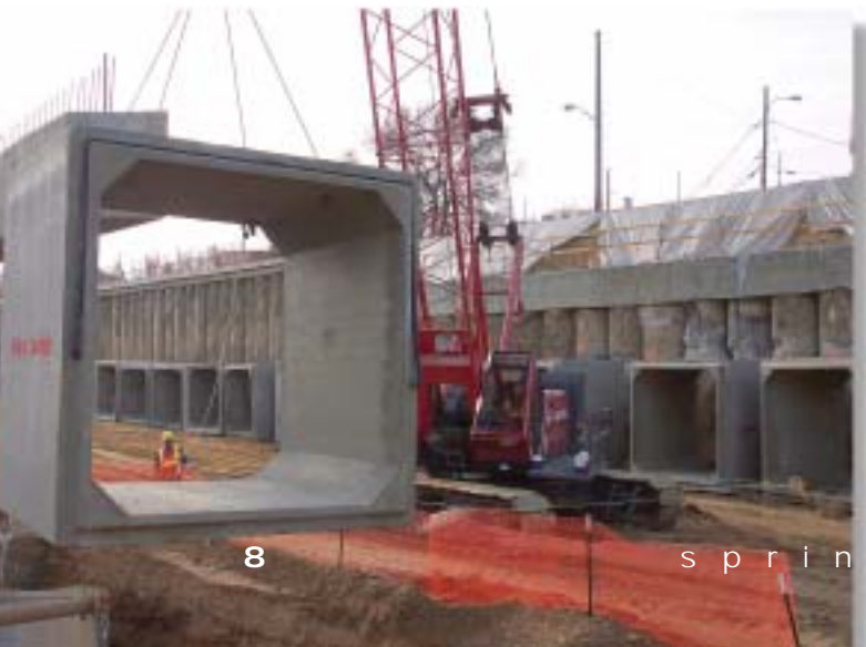
Precast concrete box sections being positioned for installation as part of Denver's T-REX Transportation Project.
