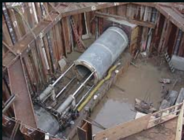
Denver's T-REX Transportation Project includes 1,500 feet of precast concrete pipe that will be bored and jacked into position.
