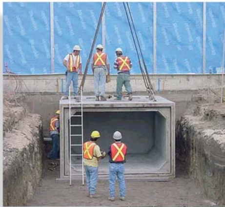
The precast concrete box sections were installed on a “mud slab.” Sand bedding was placed over the mud for leveling the boxes as they were installed.
