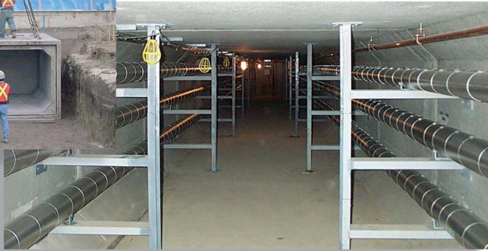
The below-grade precast concrete box structure provides excellent security and convenient access to the HVAC piping systems.
