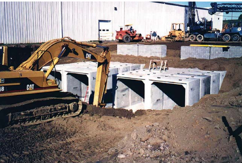
Four 8-foot x 9-foot precast concrete box sections were installed as a sub-grade building component for the building's heating, ventilation and air conditioning system.
