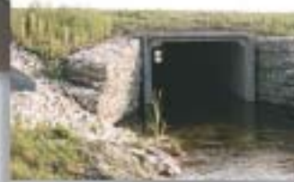
...and provide an attractive and structurally sound culvert solution under the TransCanada highway.
