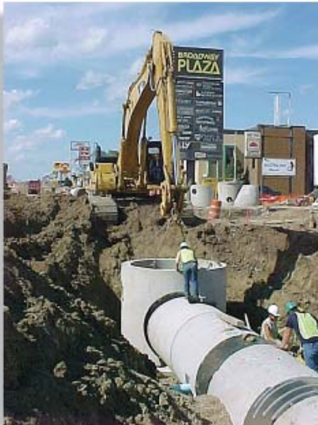
A precast manhole with integral base is connected to the 60-inch diameter RCP along South Broadway.
