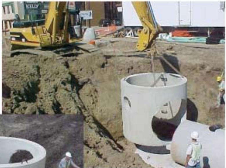
Precast concrete products were used to expedite construction and help reopen the major thoroughfare to travelers and local businesses.
