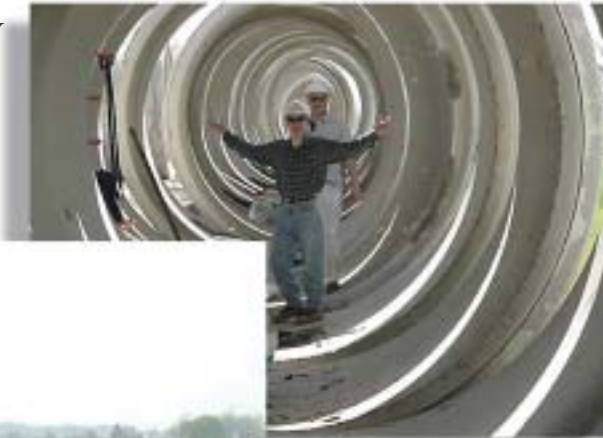
Two new parallel drain lines included Class IV RCP from 66-inch to 126-inch diameter.
