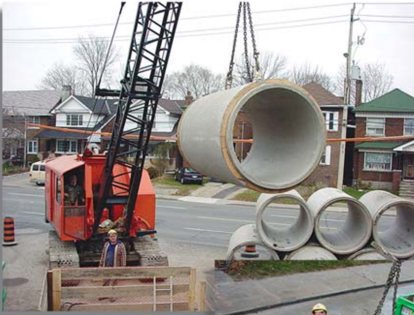
Swift Lift® lifting devices and steel bands around the pipe bells were integral components of the precast concrete pipe manufactured by Munro Concrete Products Ltd.
