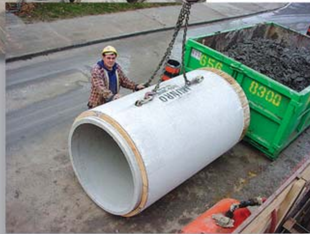
The reinforcing steel of each pipe was extended into the spigot to enhance jacking performance.
