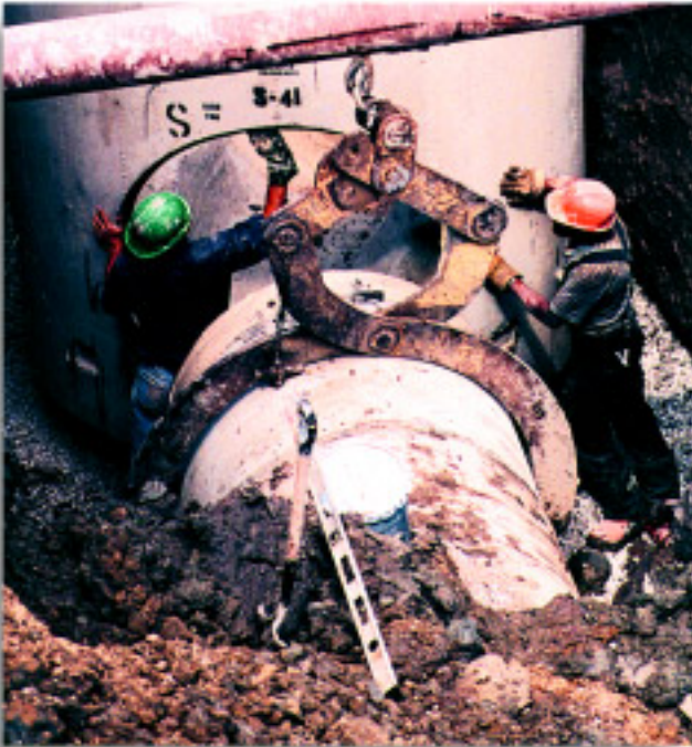
Stringent quality control efforts and exacting installation procedures yielded watertight joints at all manholes.
